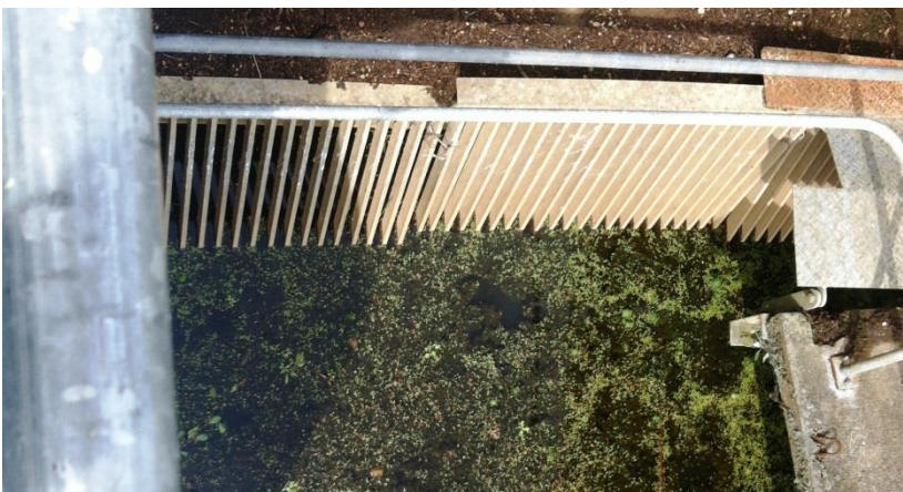
Figure 8: 50mm debris screen on Motukaraka scheme axial pump intake (photo – R. Duirs, BBO)
