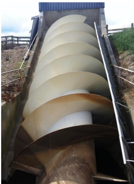
Figure 2. Motukaraka Archimedes Screw Pump (photo – R. Duirs, BBO).
