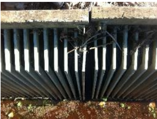
Figures 27-29: Photos of the electrical eel barrier installed at the Meremere pump station, Waikato. (Top left) view of pump station and screen. (Top right) Electrical connection on left of screen array which is duplicated on right. (Bottom left) Gap between the screen panels which insulated the left and right electrified screen panels (photos - J. Boubée, NIWA).
