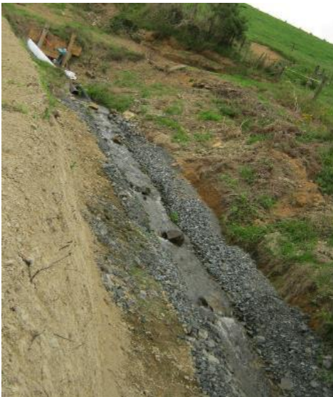
Figure 52. Open channel fish pass at Mokauiti Dam. In this case the main flow is provided by a syphon and at the end of the channel a pipe (white pipe top left) has been sunk through the embankment to allow fish to reach the head pond (photo J Boubée, NIWA).
