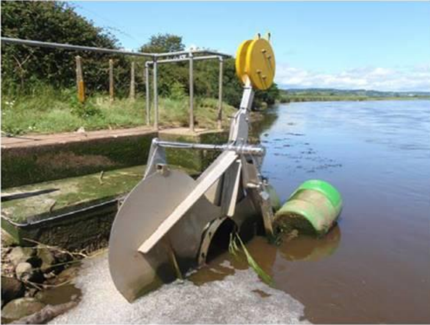
Figure 45. Guillotine style self-regulating floodgate (photo: Ridgeway & Williams 2011)
