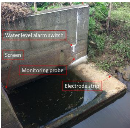
Figure 31: View of forebay - Mountain Rd pump station, Hikurangi, Northland at low flow. Voltage for the electric barrier is applied between the screen and the electrode strip that runs along the side and floor of the structure. Equipment that measure and logs the voltage between the earth strap and the monitoring probe is used to warn the operator of malfunction. At this site a water level switch has
