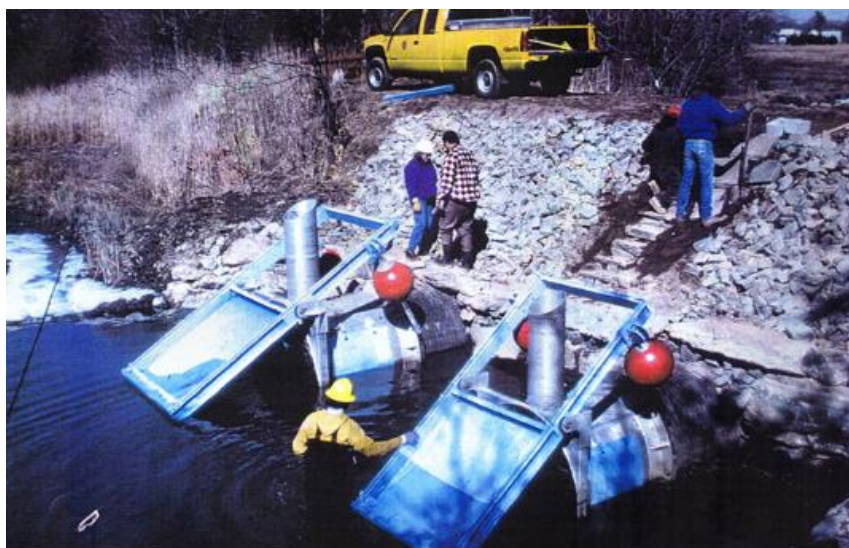
Figure 44. Installation of a Waterman self regulating tide gate in the USA. These gates close at pre-set level maximising fish passage while maintaining flooding security. (from http://watermanusa.com ).
