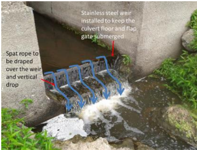
Figure 48. Modification of the Te Mata Pump Station outlet, Hikurangi Flood Scheme. (photo - from presentation to stakeholders by Adam Twose, Whangarei District Council)
