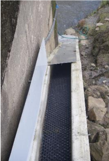
Figure 50. Fish ramp at Wairua Power Station, Northland. The open lid panel reveals the studded floor lining used as a climbing medium. The ramp in this case is concrete and the lid aluminium. (photo J Boubée, NIWA).
